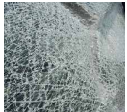
Destructions of glass in Oslo's centre after bomb explosion.
